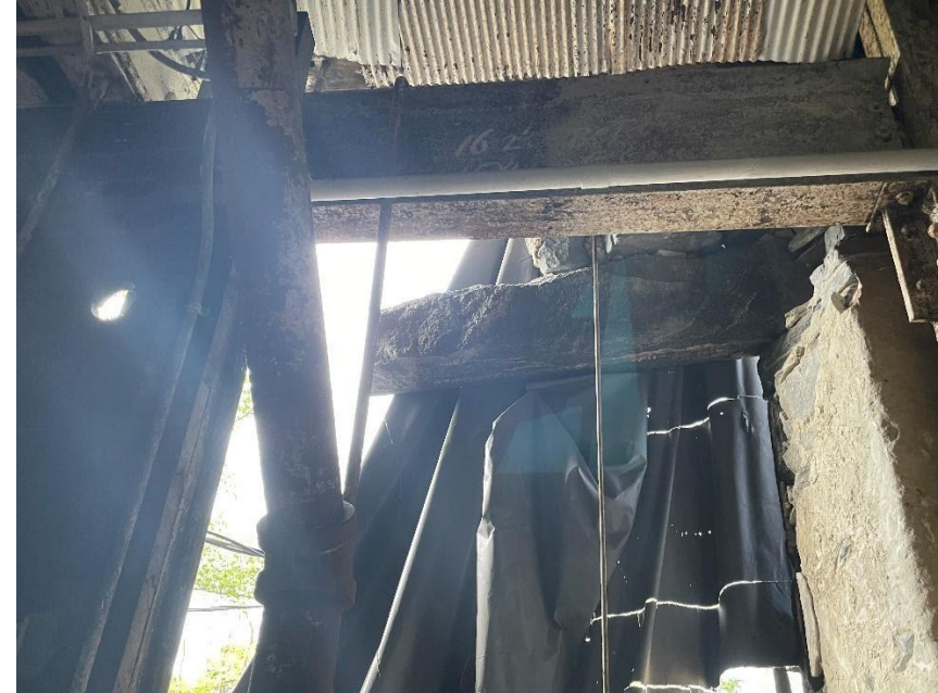
Collapsing Façade - from Interior of Granite Building
