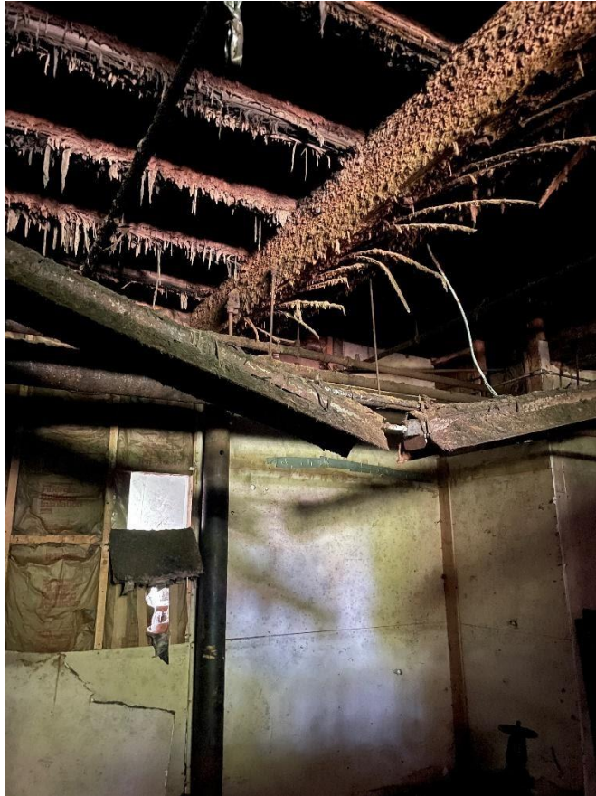
Cellar of Granite Building - Evident Structural Compromise from Water Intrusion
